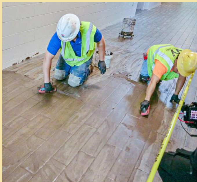
With the tiles set, the team prepares for the final step: applying Ultracolor Plus FA grout to ensure a durable, color-consistent finish that stands up to heavy foot traffic.
