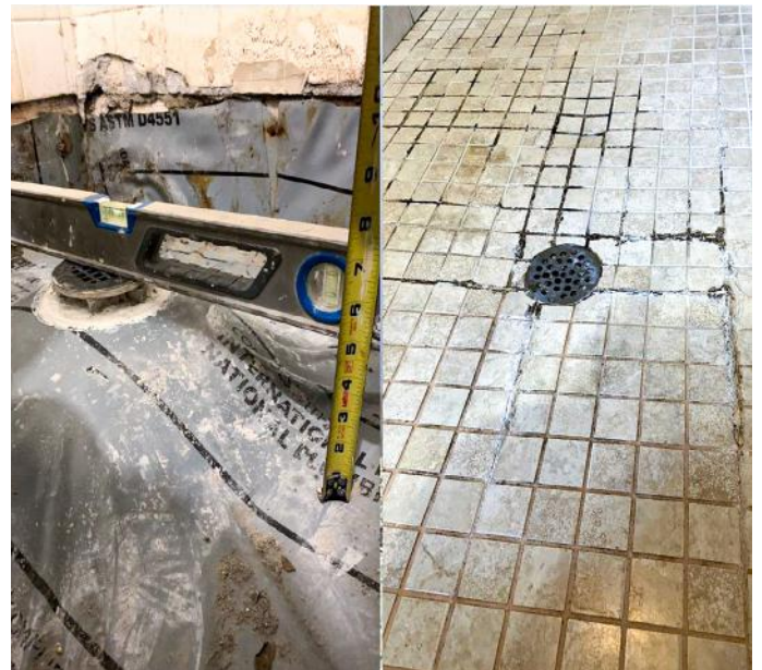
The NTCA Foundations of Wet Areas workshop aims to educate installers so they can prevent catastrophic failures in wet areas and shower installations.
