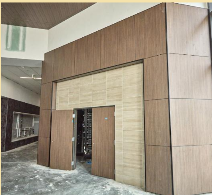
High-performance wall tile reaches heights of 24’ in the main entryway, showcasing the extreme bond strength of Keraflex SG.
