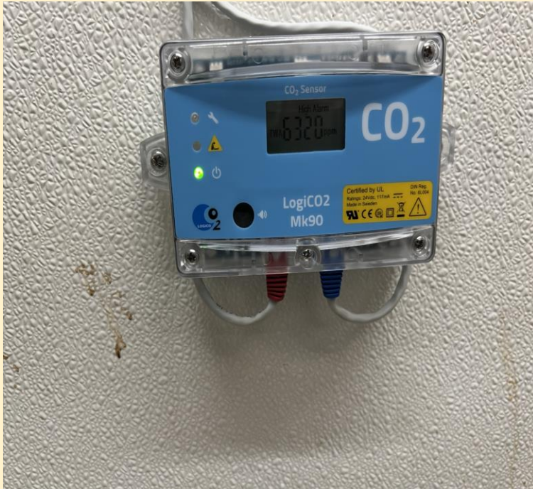
Carbon Dioxide Alarm Panel
