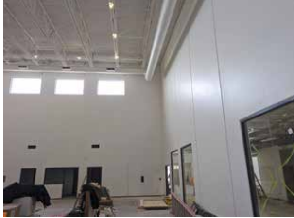
The old school was demolished in 2020 and construction on the new facility started in August 2021. It is expected to be completed in June 2023.
