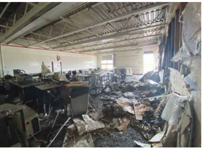
Smoke and soot, if left untreated, can cause extensive damage to both contents and structure, causing corrosion, etching, and pitting that only worsens with time.
