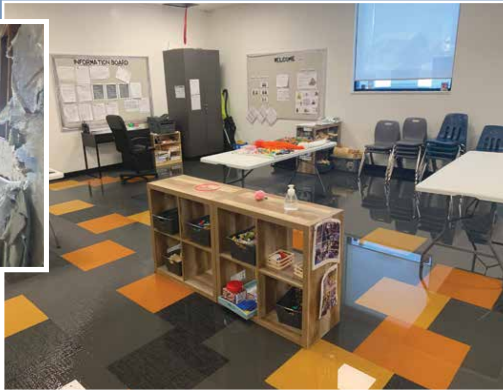
The key to minimizing water damage – whether it be from a sewer backup, burst pipe, or weather event – is a quick response.
