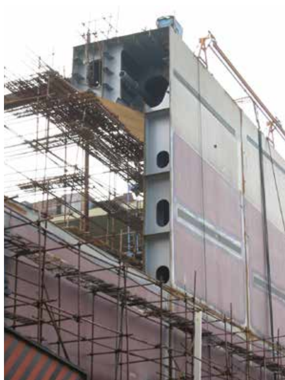
Figure 1.2 Double-skin construction. A midships hold of a Diamond 53 vessel (Both photos courtesy of Niels Bjørn Mortensen)
