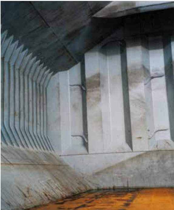
Figure 1.4 Hold of conventional bulk carrier. Anticlockwise from top left: topside tank side plating; shell plating with vertical framing; DB hopper side tank; tanktop plating; bulkhead stool; corrugated bulkhead
