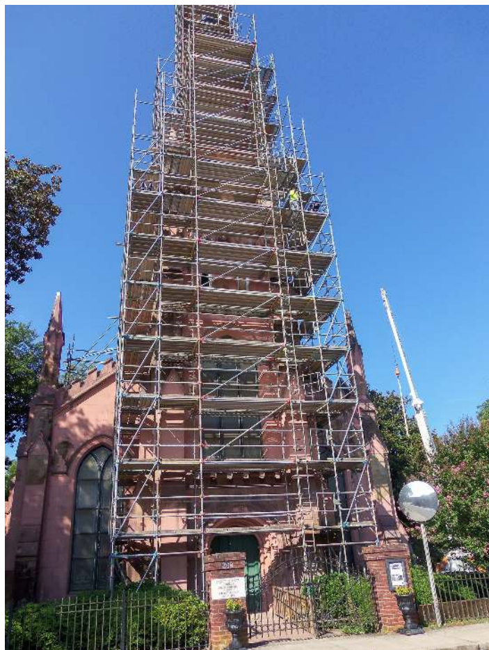
Restoration work at Trinity Episcopal Church continues, and copper liner for the drainage system around the spire is being installed, said Mike Bedenbaugh, acting president of Preservation South Carolina. (Staff photo by Henry E. Green)
