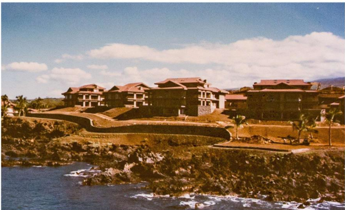
Phase II Buildings 11, 12, 13, and 14 were prepped for landscaping. A huge retaining wall along the Ocean Walk was complete. Nov 1986
