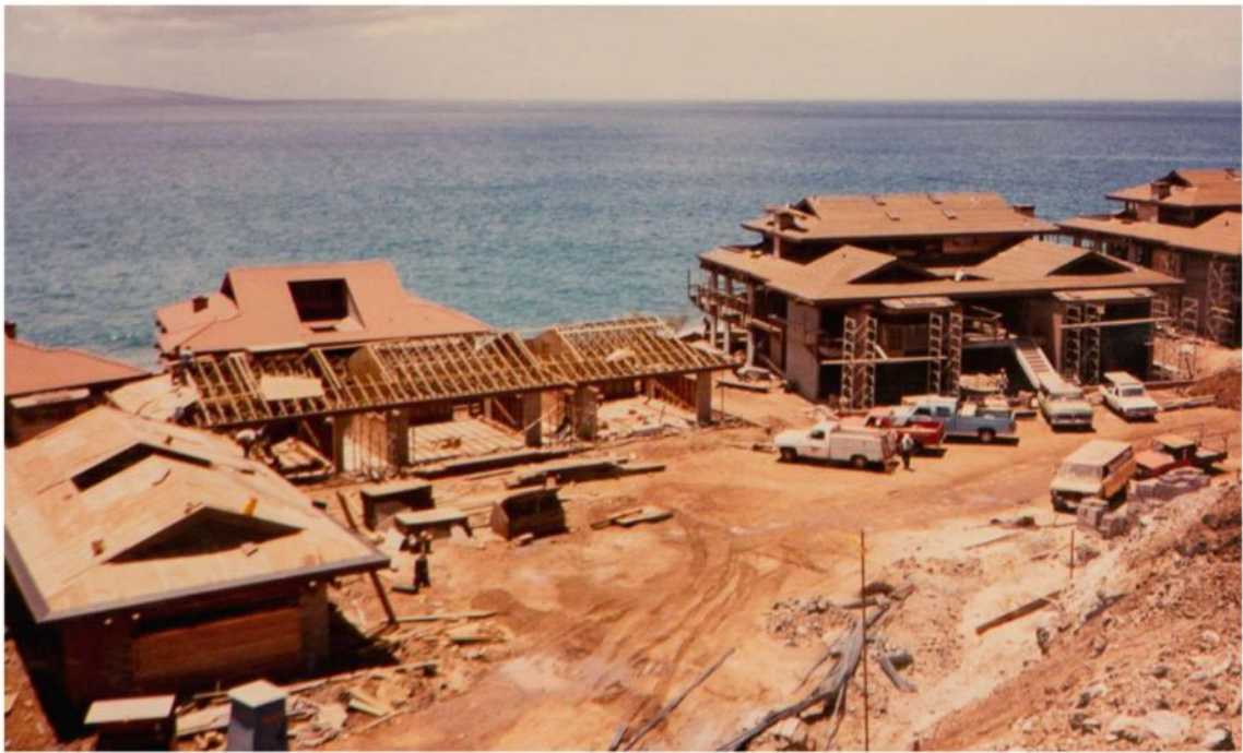
At the south turnaround of Phase II, workers' trucks parked in front of Building 15, the roof was already on Building 16, and car garages were underway. Aug 1986
