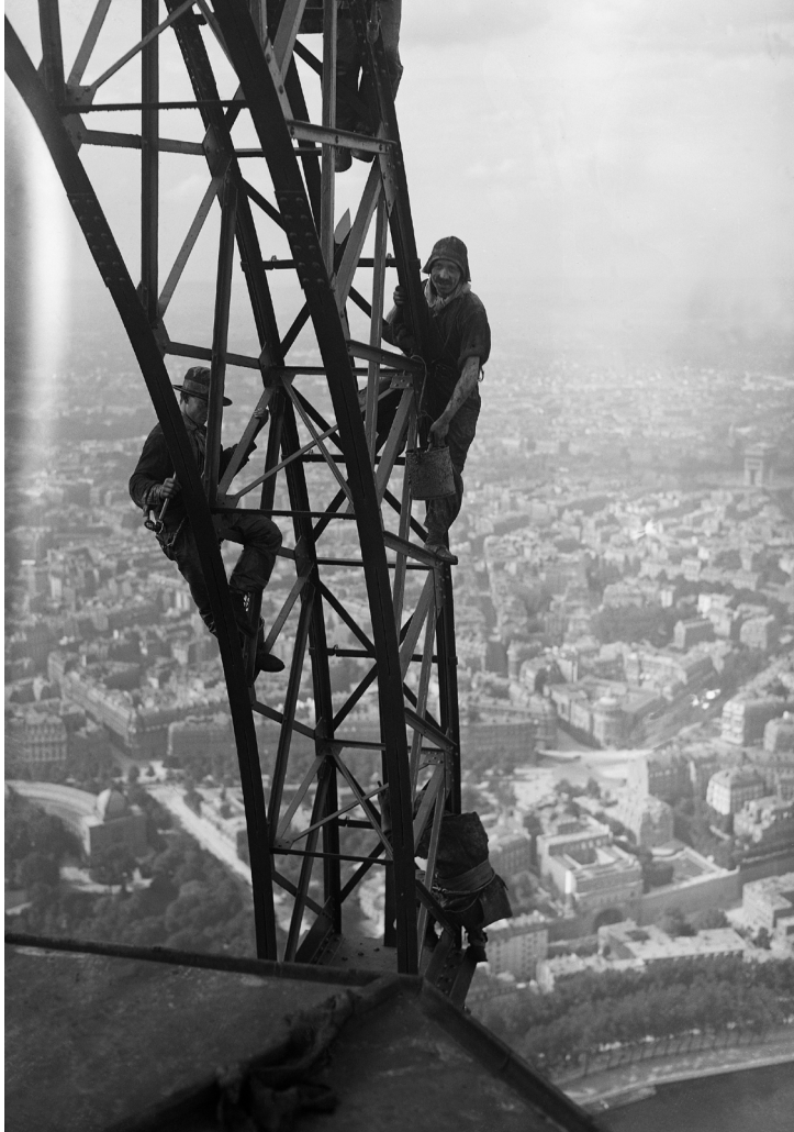
'Like some fabled city descending to the bottom of the sea': the view of maintenance workers on the Eiffel Tower in 1924.
