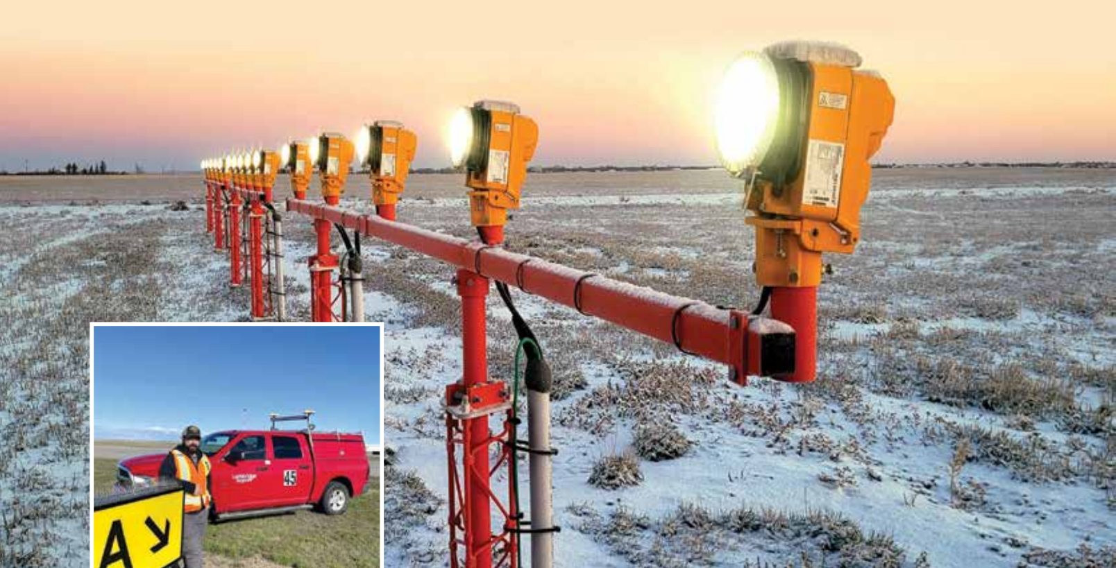
Above: The design of airfield circuits—built around a series current-driven model—makes the systems not only dangerous, but also more difficult to repair. Inset: Anthony Kish, an experienced airfield electrician at the Lethbridge Airport.
