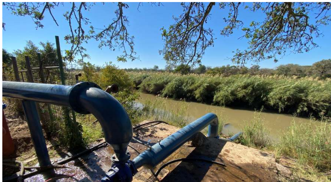
Pump station on the Klaserie River
