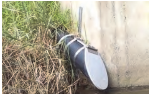
This pipe, unfiltered, brings water from South Shores into the Bungala estuary. The water builds up at South Shore; when it gets to a certain level, a pump then pumps it straight into the Bungala estuary. (It's believed flooding is caused from a leak in the lake at the Links.)
