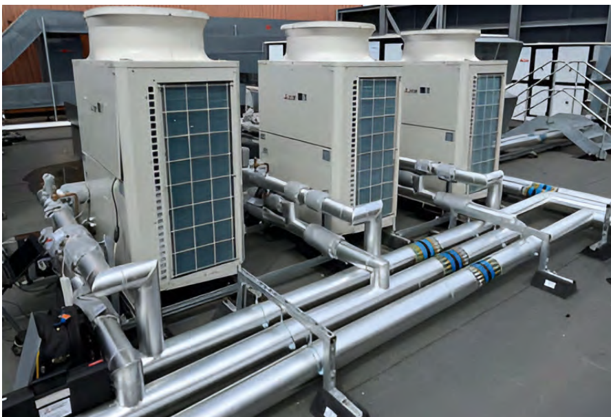
Commercial heat pump installation with metal clad pipework, installed by a thermal insulation contractor
