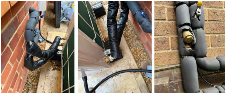
Insulation of heat pump pipework is often an afterthought for heat pump installers
