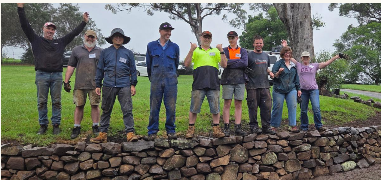
Junling Wang (3 rd from left) celebrates with fellow participants after completing a retaining wall at one of Geoff Duggans Walling workshops held in Picton, NSW
