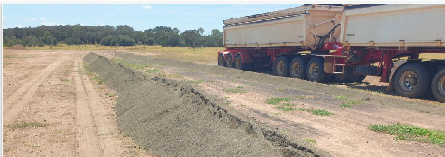
76 tonne of crusher dust being delivered with an AB double road-train (Three trailers) As can be seen, the grass has started to grow through the Geofabric due to the rain.
