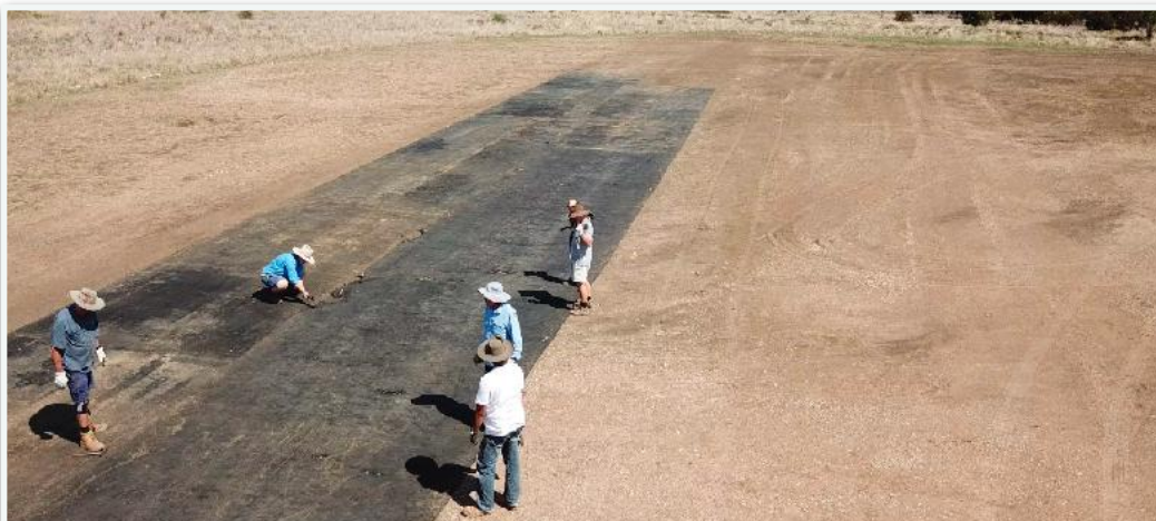
The team re-laying the Geofabric over the black soil area. About 200 mm of black soil was relocated to the area in the top right of this picture.
