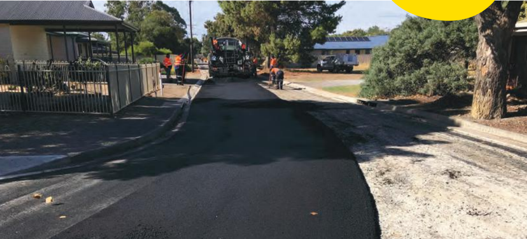
Images Above Laying the soft plastics bitumen surface on Herbert Street in Normanville.
