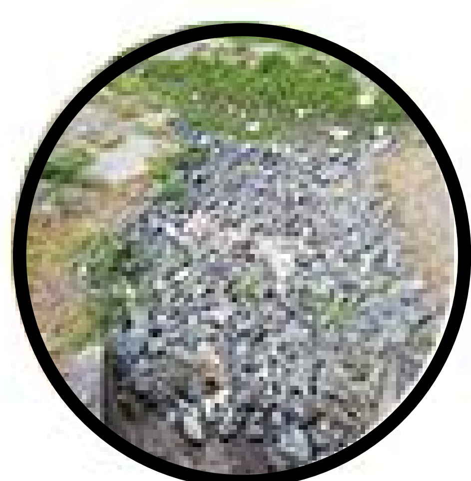
Rip- Rap water dissipater
