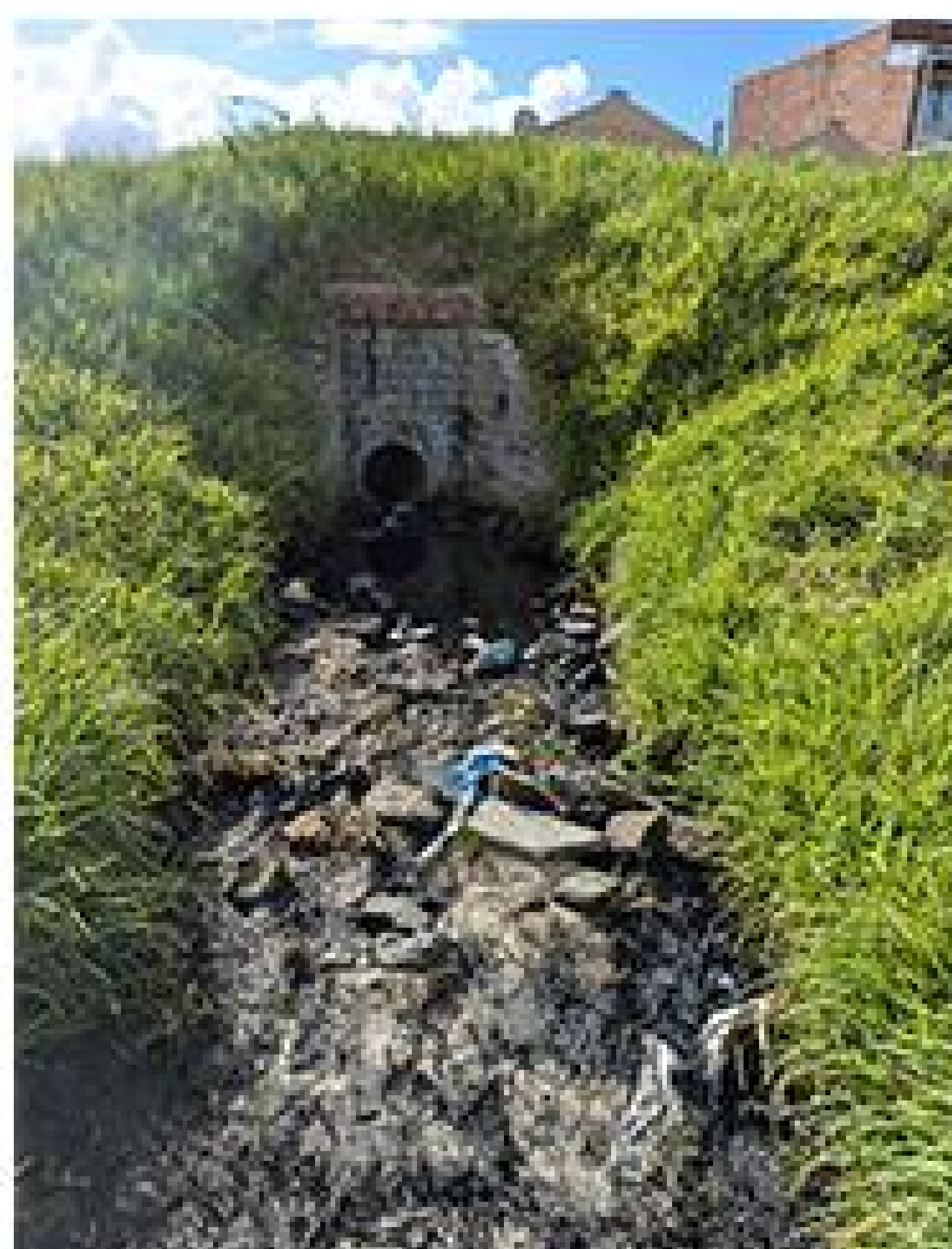
Oil spill leaks
