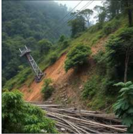
A cableway tower on an unstable slope in extreme rainfall — not a hypothetical risk.
