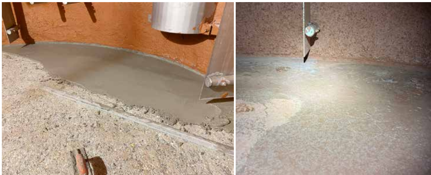
Above left: Lajcon Distributors delivers engineered, specified solutions that help mining operations preserve critical infrastructure, reduce lifecycle costs, and maximize operational uptime. Right: Dissolver tank after three years.
