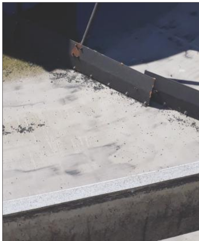
Scraper blades after the tank was drained following a year's service.
