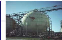
◀ Liquid level monitoring of oil storage tanks to avoid overflow or leakage
