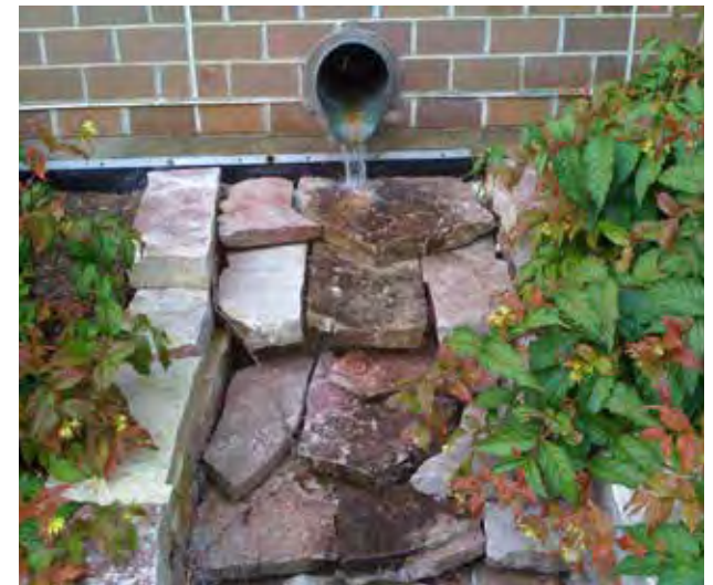
Figure 5.38 Exposed Water Draining from a Rooftop. Copyright: Conservation Design Forum
