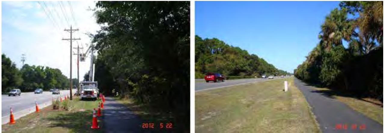
Figure 5.21 Before (left) and After (right) the Burial of Overhead Utility Lines. Source: Scenic America, Hilton Head
