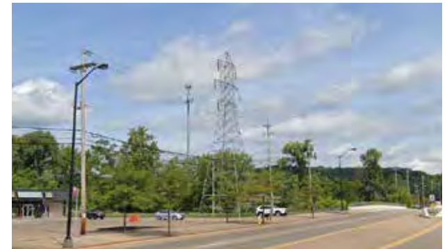
Power lines and Pylons
