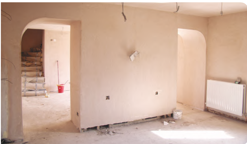
Preparation Phase: First fix successfully finished, setting the stage for the laying of the floor, decoration & the arrival of the new kitchen furniture.
