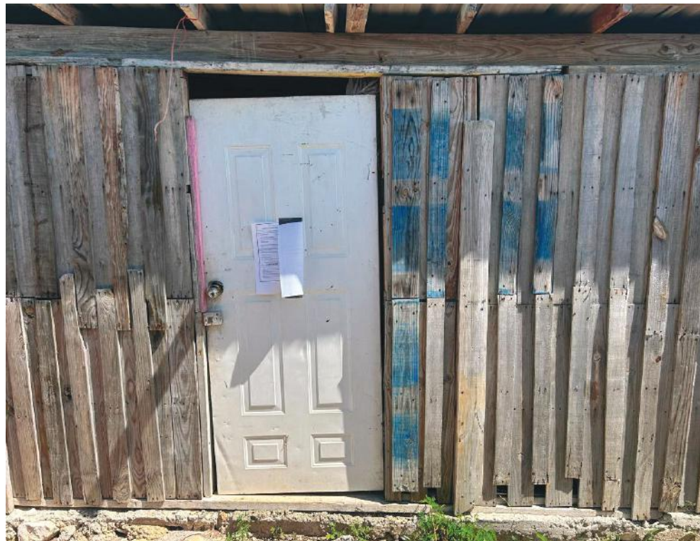
A notice of demolition is affixed to a structure by the Informal Settlements Unit
