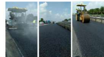
Photos of 1 st Field Trial at North South Expressway South bound, Fast lane (June 14, 2017)
