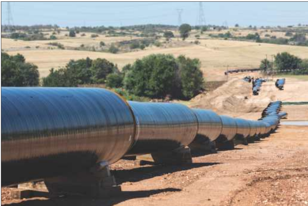
Protecting critical infrastructure against corrosion remains a maintenance issue but a business imperative to keep operations steady and costs low.
