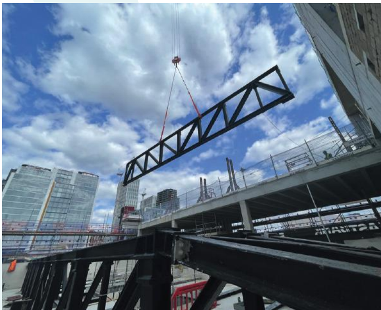
Above: A section of the steelwork destined for the main dance studio being lowered into place
