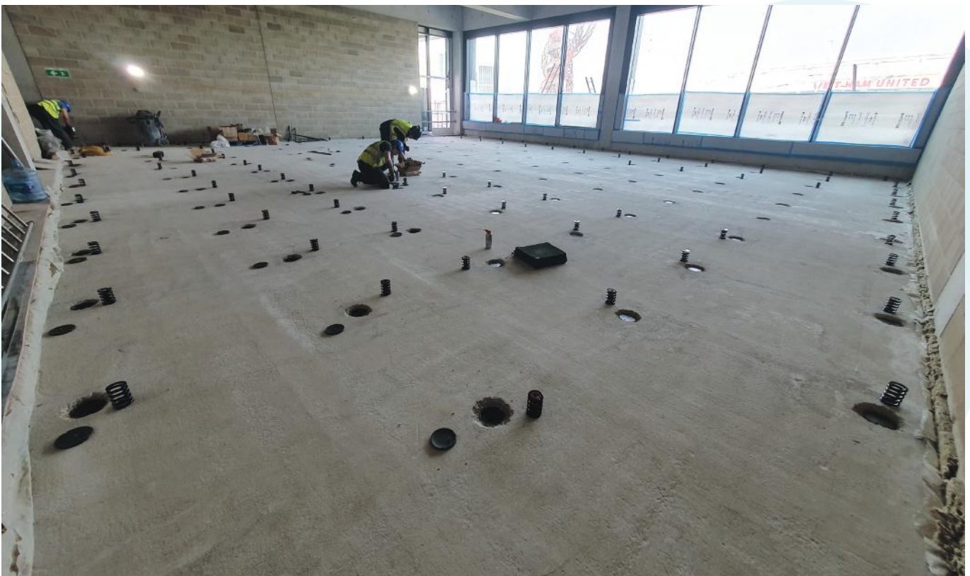
Above: Inserting the floating floor springs before commencing jacking, to within 5mm across the whole area
