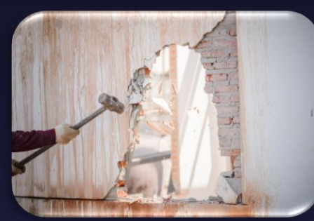
Wired solution damages walls
