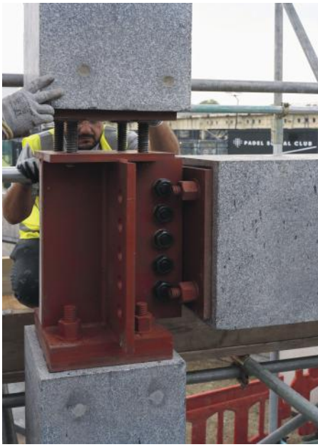
Above and right: The Stone Demonstrator by Groupwork with Webb Yates and Arup features pre-tensioned stone beams and columns, linked by steel tendons.
