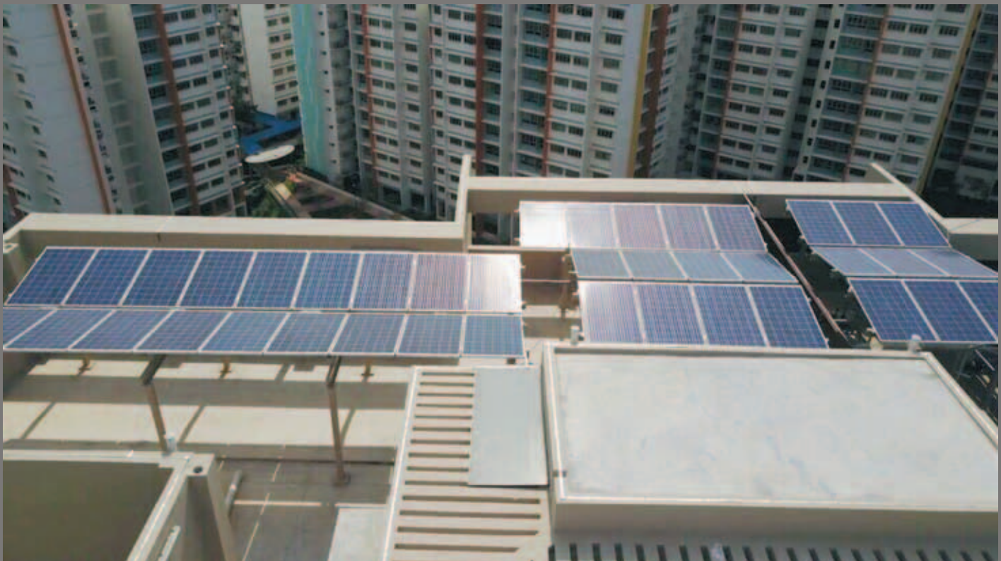
Photovoltaic Panels Elevated from Roof Floor
