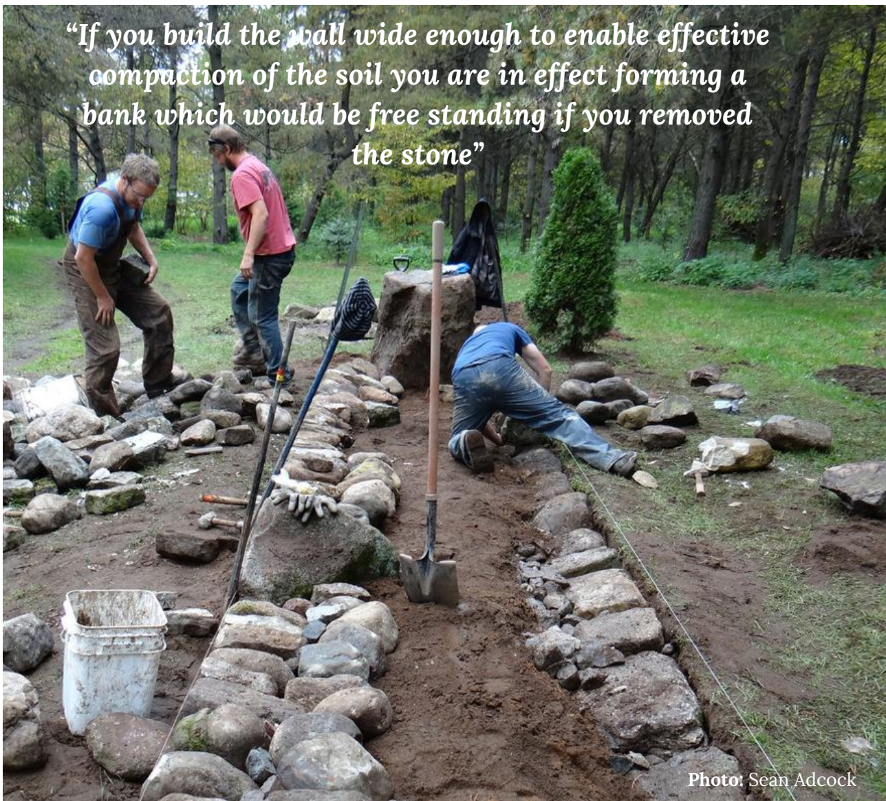
Participants in a Canadian workshop building a clawdd foundation. The double 'skin' of foundation stones is intended to ameliorate frost heave.
