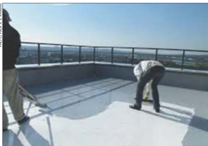
Special waterproofing materials are used during initial construction that can take care of leakages throughout the life of a structure.
