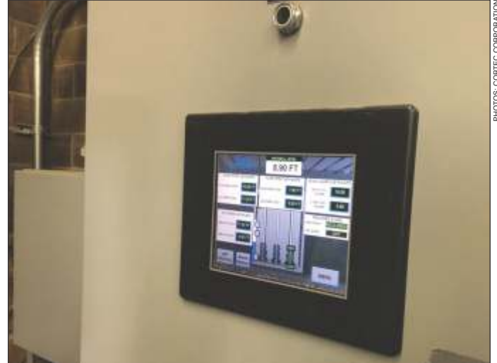
A Midwest US wastewater treatment plant used Cortec® corrosion solutions to halt the failure of expensive HMI (human machine interface) panels at the rate of one or two every six months.
