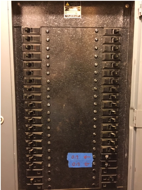
Figure 2: A 200-amp electrical panel, also called a breaker box.
