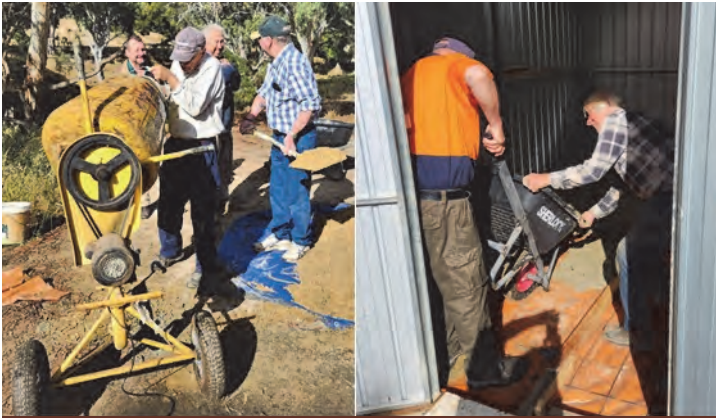
February 3rd 2023 making cement for new floor; Laying cement on new shed floor
