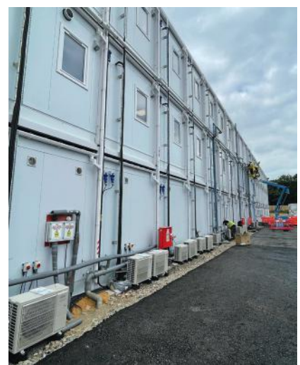
To date, 82 systems have been installed with 20 more to follow
