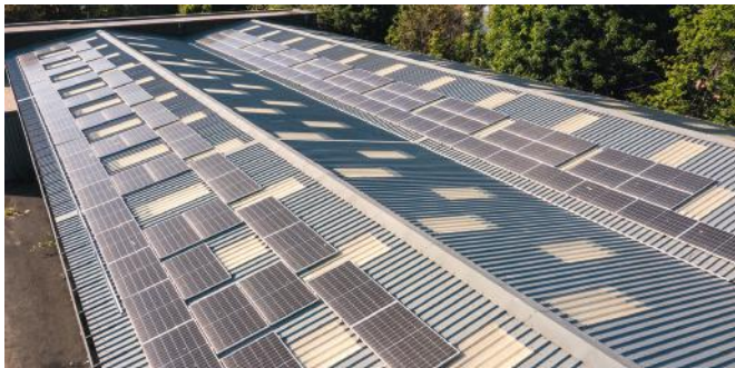
Solar PV panels on the rooftop at CDL's Gateshead headquarters
