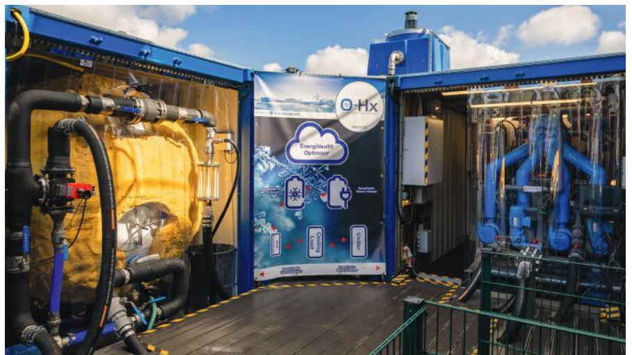
The patented EnergiVault cold thermal energy storage operating at Quotient Sciences, Alnwick
