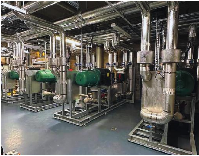
Four Gorac refrigeration packs, based on BITZER screw compressors, maintain perfect ice conditions at the new ice centre
