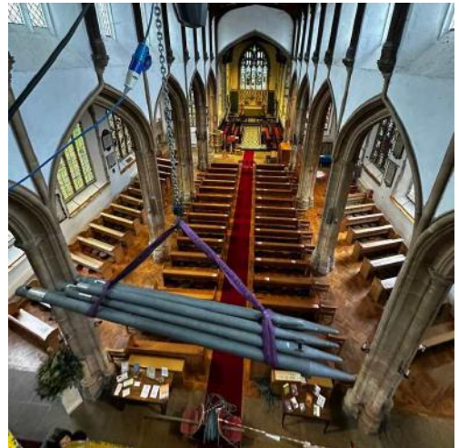
Looking down the Aisle from the platform with a load of pipes ready to be lowered to the floor.
