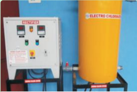
CHLOROGEN - ON SITE CHLORINE GENERATOR
