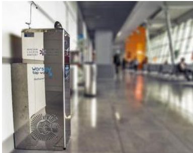
Stations de distribution d'eau (Source: Smart Water Magazine)
