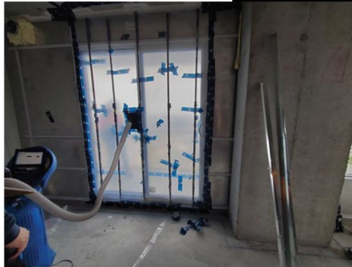
FT.01.04.C - View of interior test chamber.
