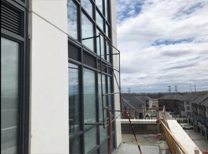
FT.01.02.A - Outside Suite 409: View of spray rack on the slab bypass area between level 3 and level 4.
