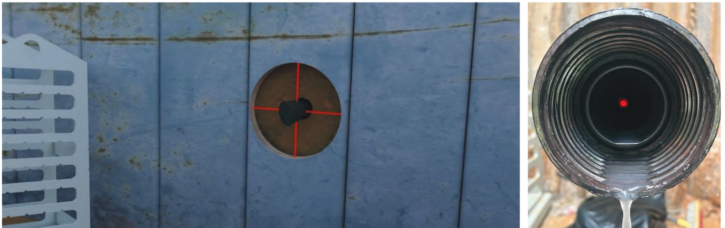
Figure 3: Photo of steering head in reception shaft and view of target (naked-eye) of installed pilot tubes at 300-ft.
