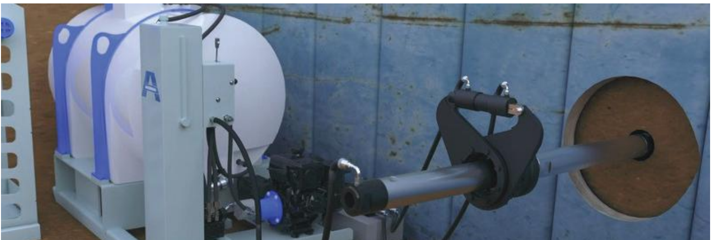
Figure 4: Illustration of the Akkerman pilot tube break-out tool, lubrication system, and air/fluid adapter setup in reception shaft. By threading on the air fluid adapter to the last pilot tube, lubrication can be added from the reception shaft, through the pilot tube string to the cutter face to reduce jacking forces and assist in processing the material.
