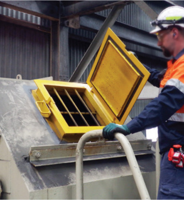
Chute Access Doors
