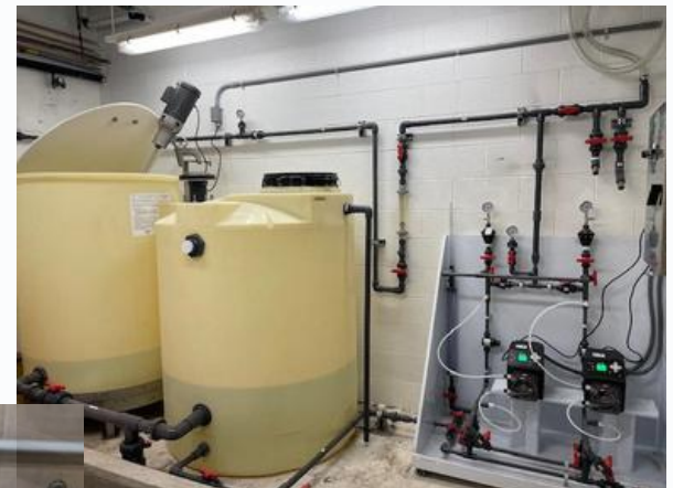
New Soda Ash Chemical Feed System
