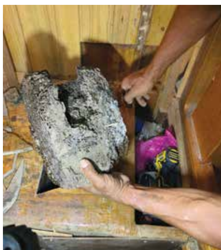
Termite nest inside the water tank
