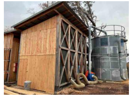
Biomass boiler system outside
